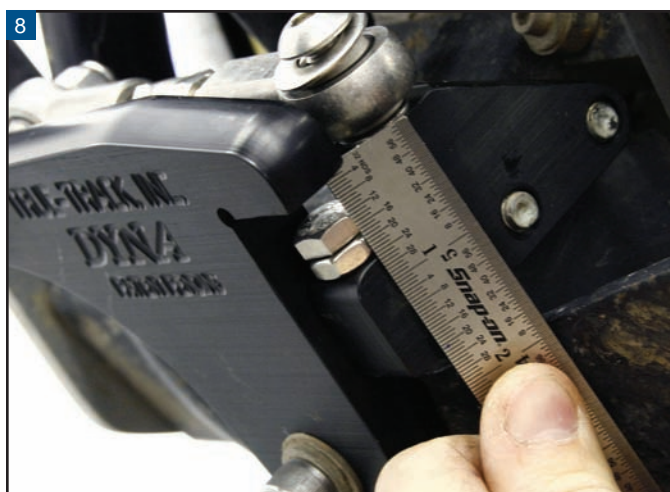
Adjust the stop-bolt on the powertrain bracket to measure 3/8" between the bolt head and the frame bracket.
